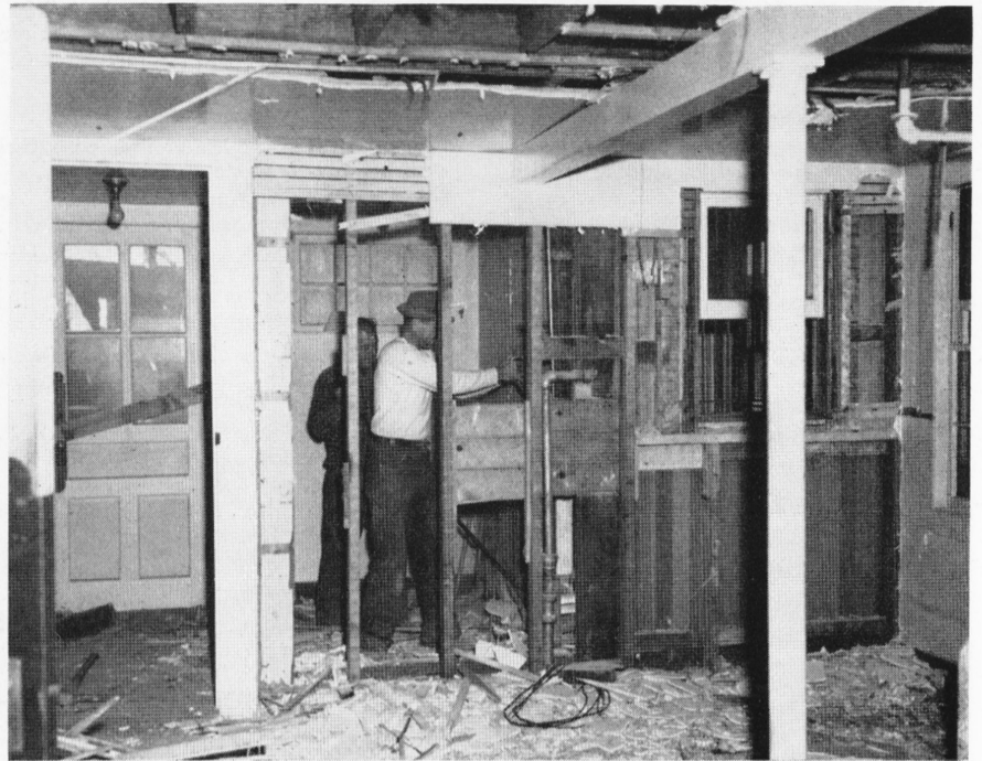
Remember the old Employment Office Building that the Credit Union just evacuated? Well, that's going to be the new Girls' Club Rooms. Workers are all ready tearing up floors and tearing down partitions and what not to get the place all in order for the gals. Working on the job are Nick Callini and Tony Santore of W. J. Megin, Inc.
